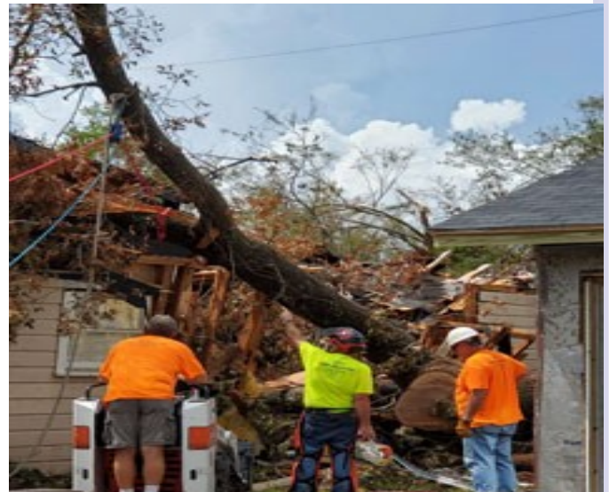
Removing tree from damaged house
